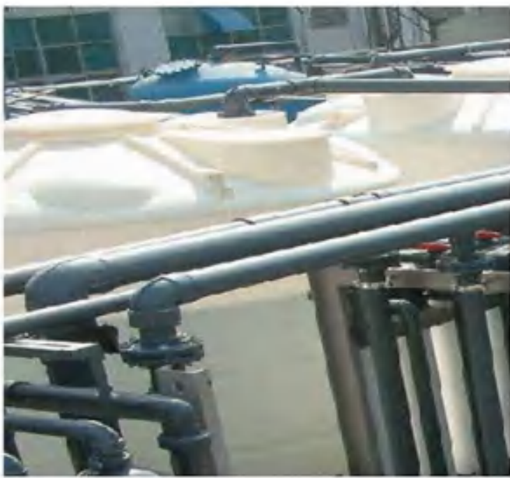
Membrane filtration MVR concentrated water to crystallization
