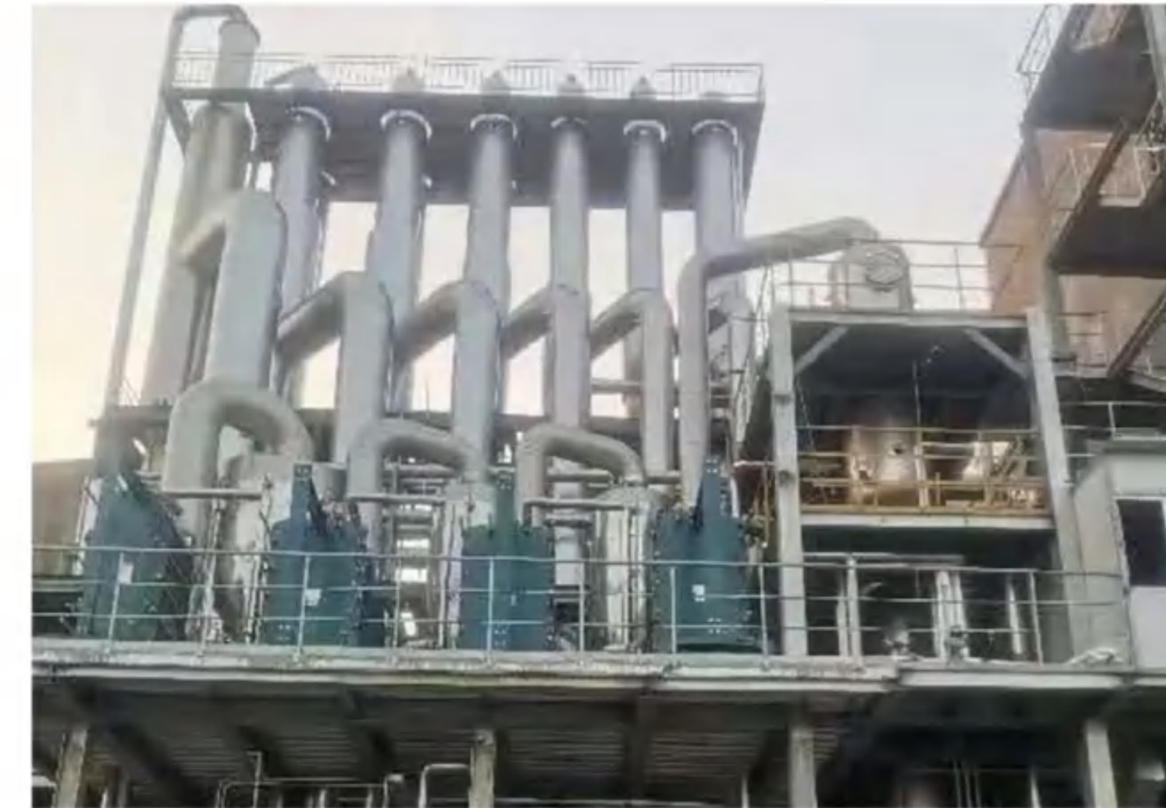
Evaporation capacity: 15.8t/h Evaporation process: triple effect plate+single effect tube Material: Potassium dihydrogen phosphate Final concentration: 60% Main material: TA2
