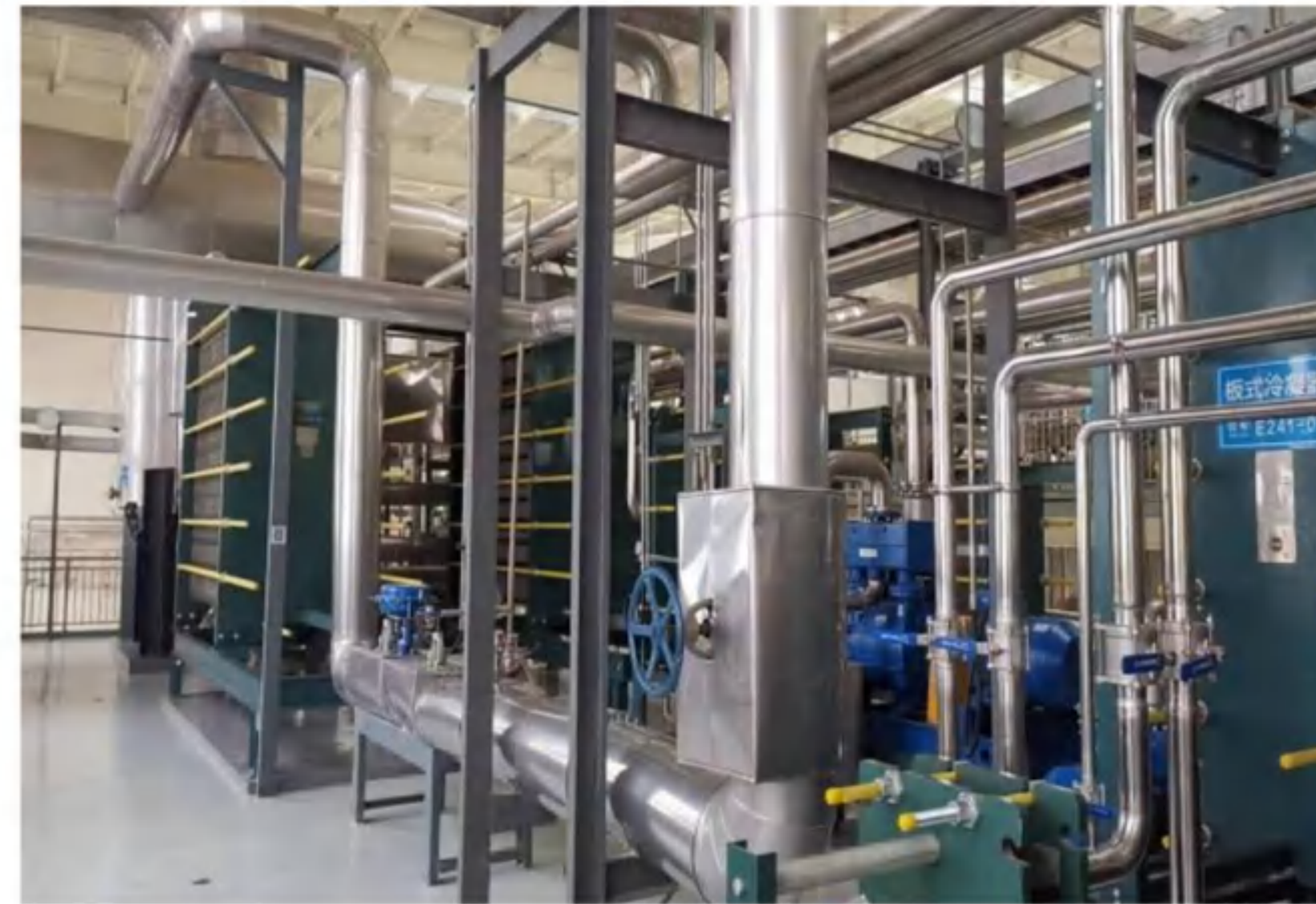
Evaporation capacity: 28t/h Evaporation process: MVR plate evaporation system Fluid: Erythritol Main material: 30403
