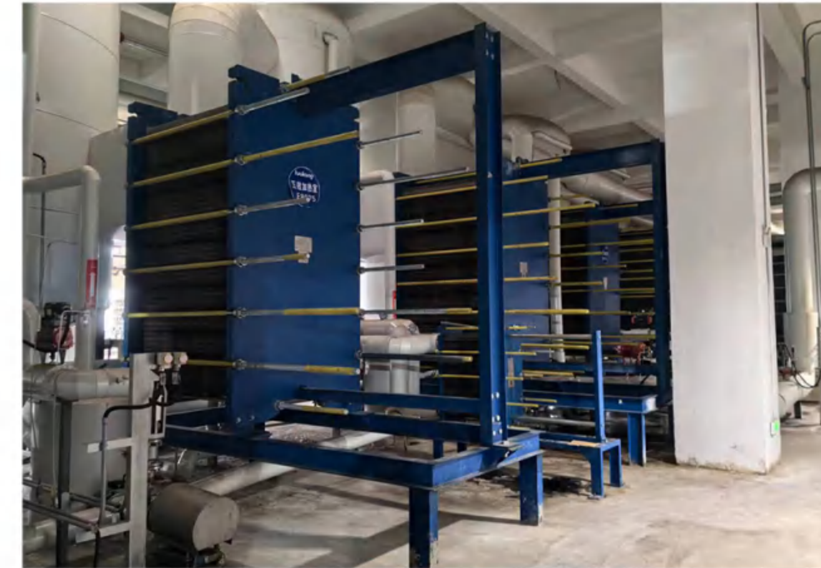
Evaporation capacity: 26t/h Evaporation process: Five effect TVR evaporation system Fluid: Xylose Discharge concentration: 50% Main material: S31603
