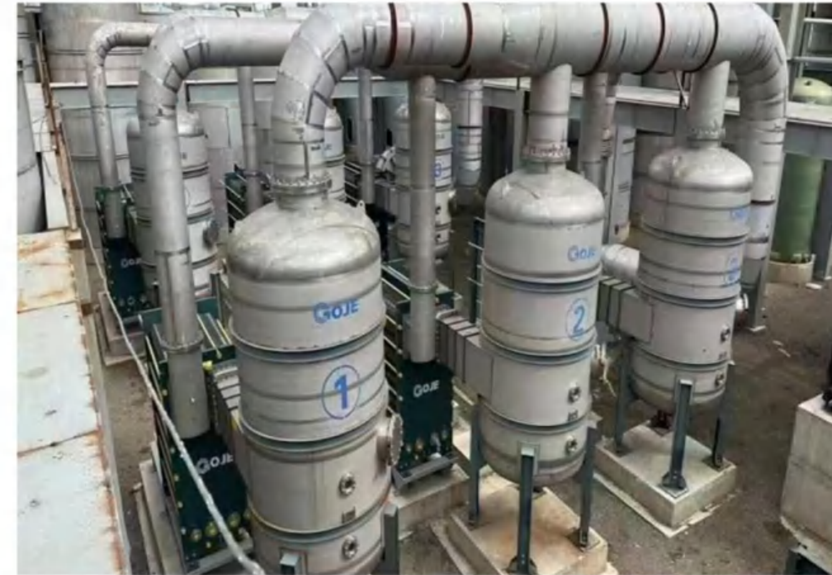
Evaporation: 20t/h 4sets Evaporation process: MVR three-effect plate Ingredients: citric acid Discharge concentration: 62% Main material: S31603
